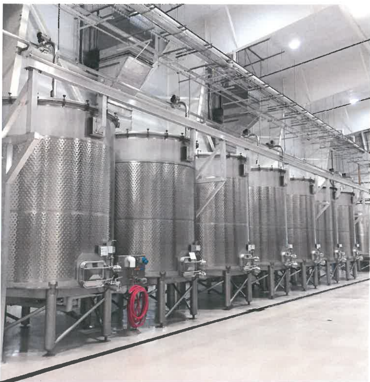
The winery has 10 open-top fermentation tanks by Santa Rosa Stainless Steel.
