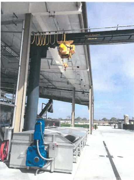
A large crane and auger are used for the largest grape deliveries to the winery.
