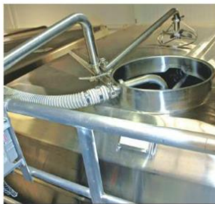
A "toad" irrigator was installed inside the truncated manway at the top of the tank to perform a 20-minute pump over supplied by a 2-inch air pump three times per day.
