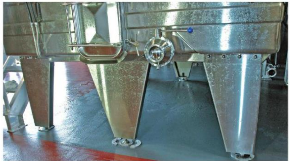
Anchor-collars surround tank feet to minimize seismic movement in an earthquake.
