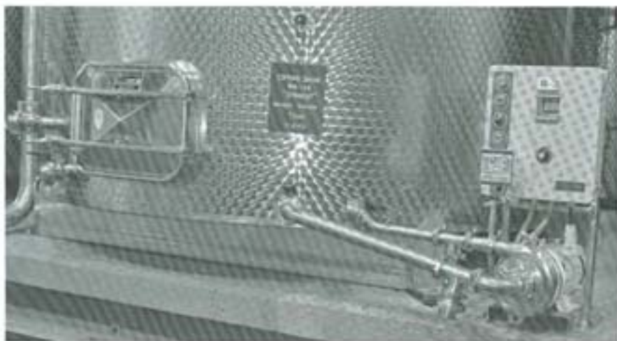
Dedicated Waukesha centrifugal pump fitted to each tank provides gentle flow of juice at 60 gallons per minute.
