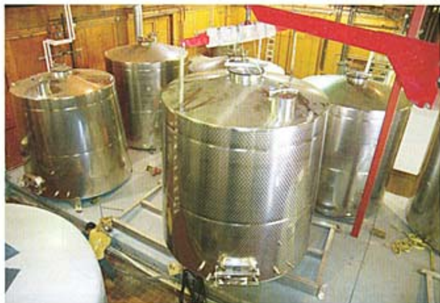
One of four new truncated tanks is placed by crane onto the tank pad. Photo by Fred Lyon.
