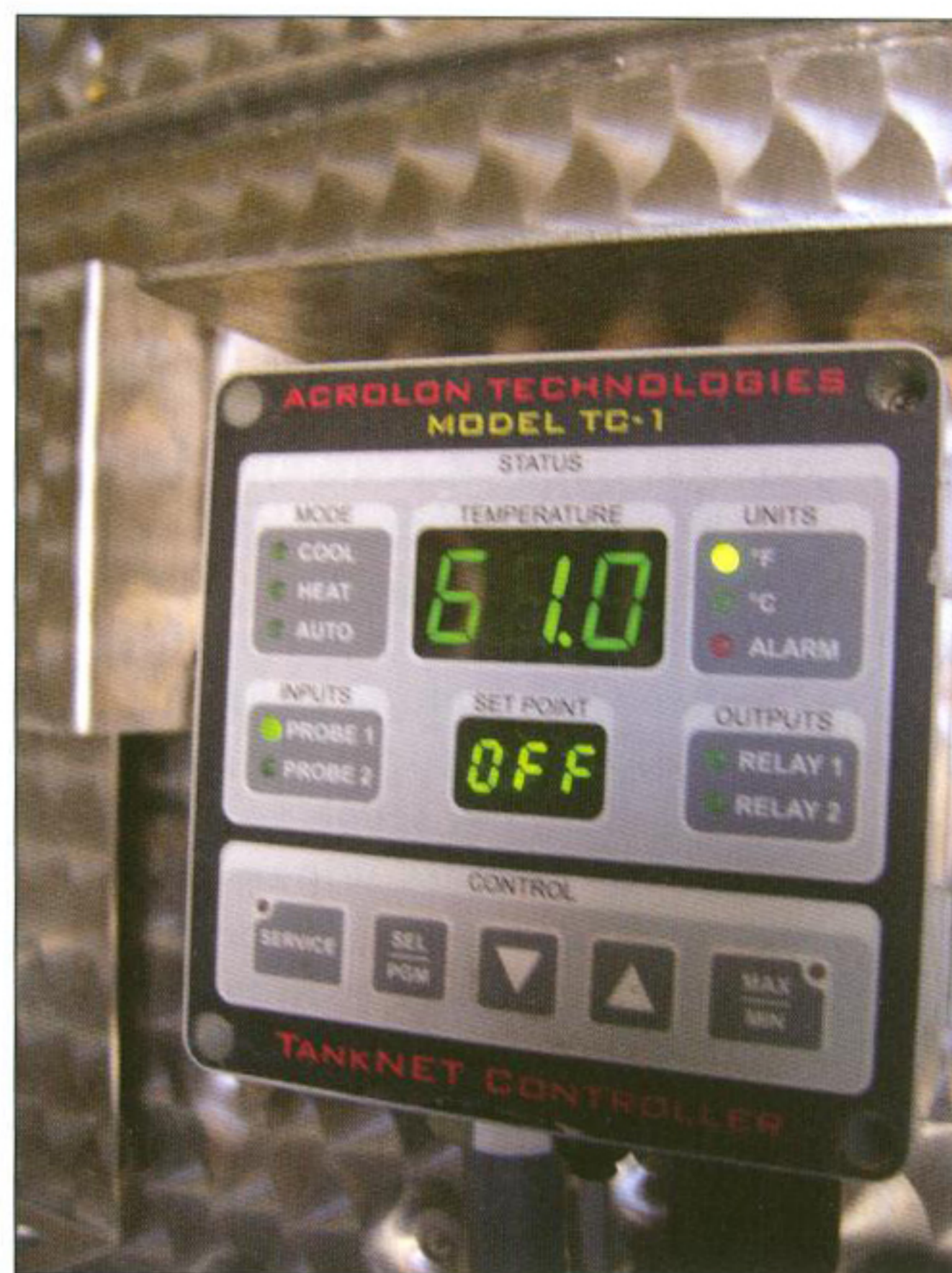
Example of a TC-1 Tanknet Controller designed by Sonoma County-based Acrolon Technologies, attached to the new open-top fermenters used at V. Sattui and Castello di Amorosa wineries.
