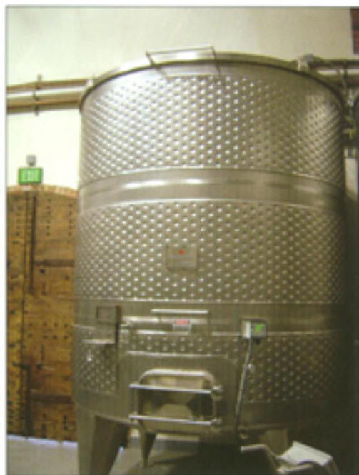
At Castello di Amorosa, one of the new Sirio Aliberti open-top fermenters equipped with a TC-1 Tanknet Controller designed by Sonoma County-based Acrolon Technologies.
